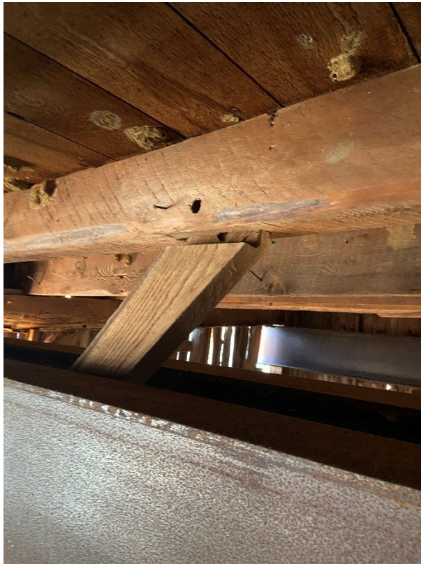
Photo 11 – Note displacement of brace from joist (exposed tenon).
