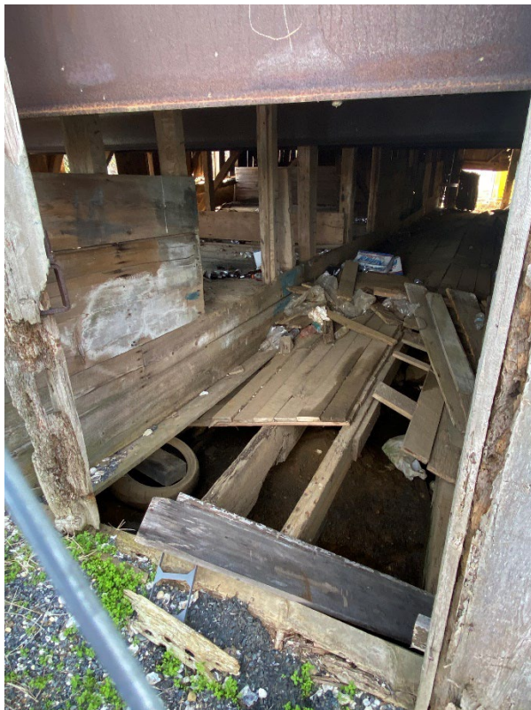
Photo 8 – Deteriorated framing at ground floor.
