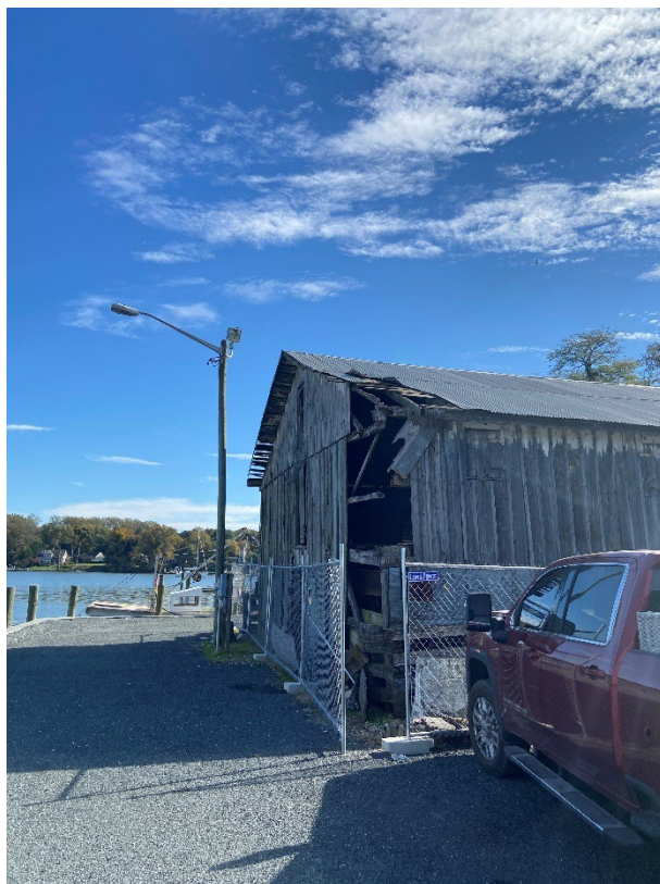
Photo 4 – Hole at northwest corner.
