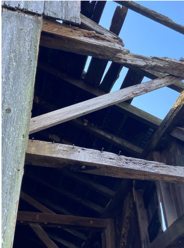
Photo 5 – Deteriorated wood framing at northwest corner.
