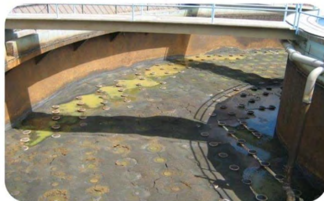
Grit Deposition in Process Basins
