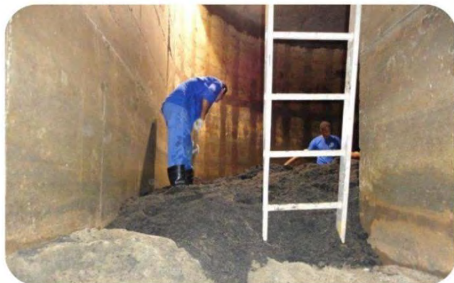
Grit Build Up in Digesters
